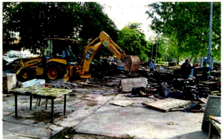
An excavator was used to demolish the stalls in Taman Saujana Puchong.
